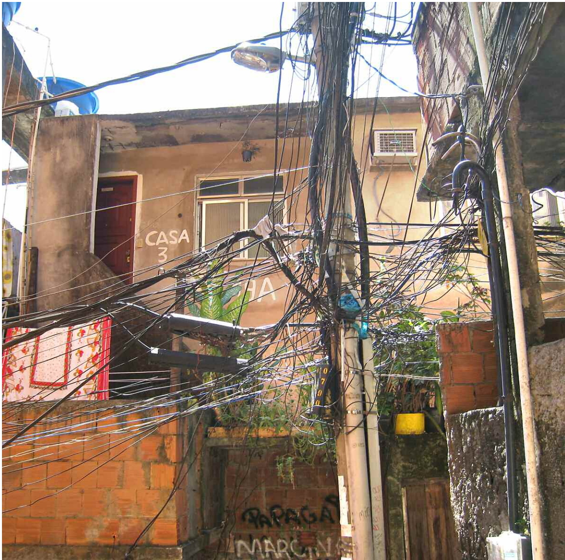
Illegal grid connections in Rio de Janeiro's Rocinha favela illustrate the demand for adequate and affordable energy (Photo credit: Alicia Nijdam)
